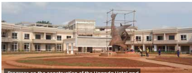
Progress on the construction of the Uganda Hotel and Tourism Training Institute (UHTTI)
